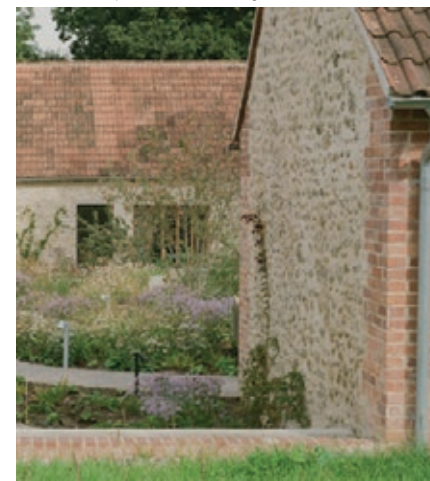
Fig 54. Sensitive gutters - to prevent further water damage
