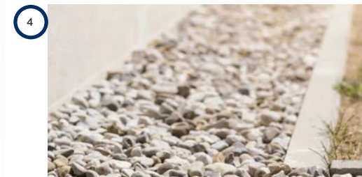
Fig 36. (4) Address damp ingress - landscape options considering soft margins or french drains to perimeter.
