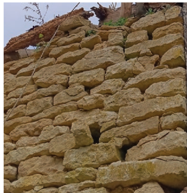
Fig 27. Loose Stonework where mortar has been washed out, March 2025. The stone itself is not generally in bad condition, and can be consolidated and re-used.
